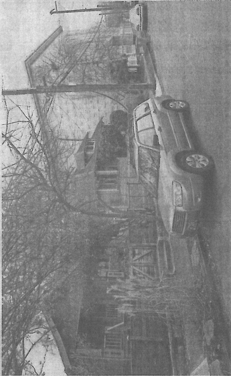
A four-story, 81-unit apartment building under construction at right shares a quiet side street with older houses in Portland, Ore. The unit will include scores of bicycle racks but no parking spaces for cars. DON RYAN/AP
